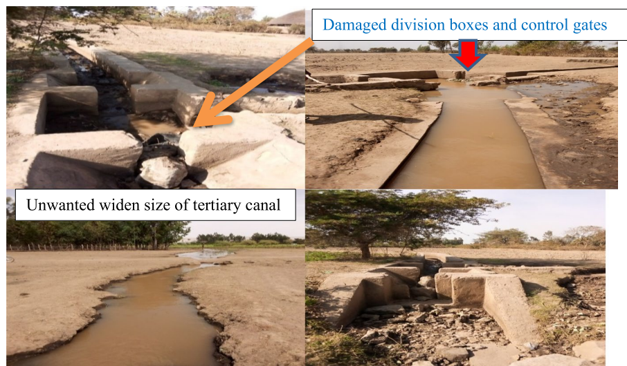
Fig. 1 Current conditions for physical infrastructures in Bilate irrigation scheme
