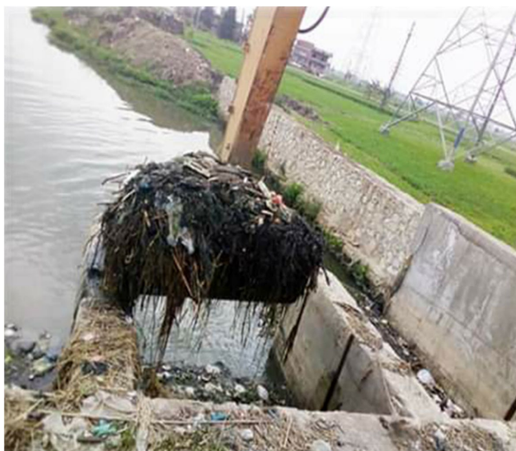
Fig. 2 Municipal waste accumulation at the entrance of a coverage structure [12]
