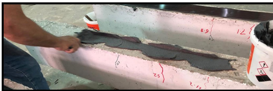
Fig. 2 Apply one layer of the epoxy adhesive on the surface of the substrate
