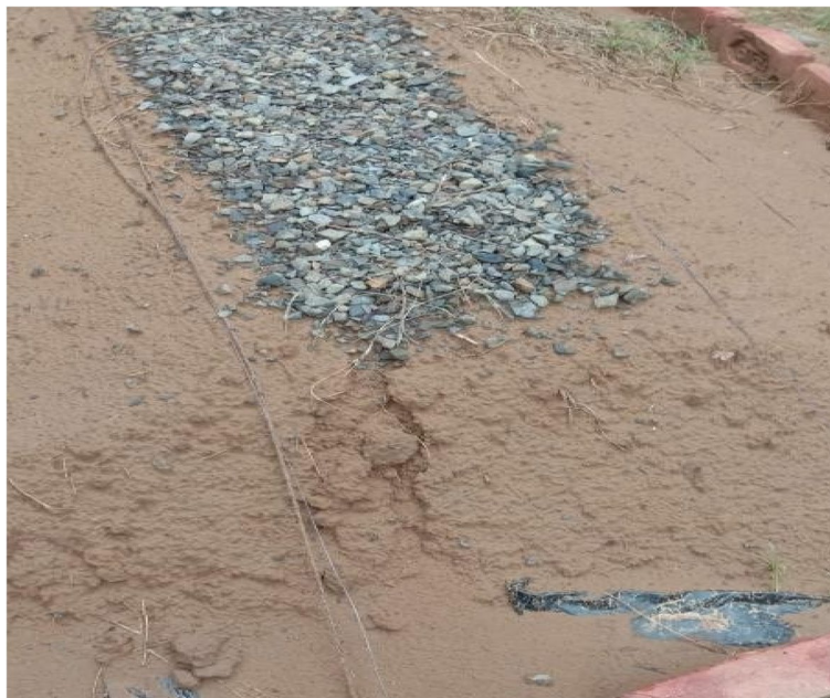
Fig. 14 Shows gully formation at less compacted central face of embankment
