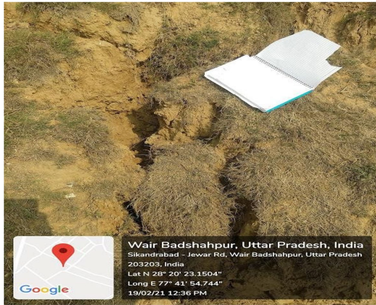
Fig. 6 Studied embankment at Wair, showing effect of gulying and slope failure no 4
