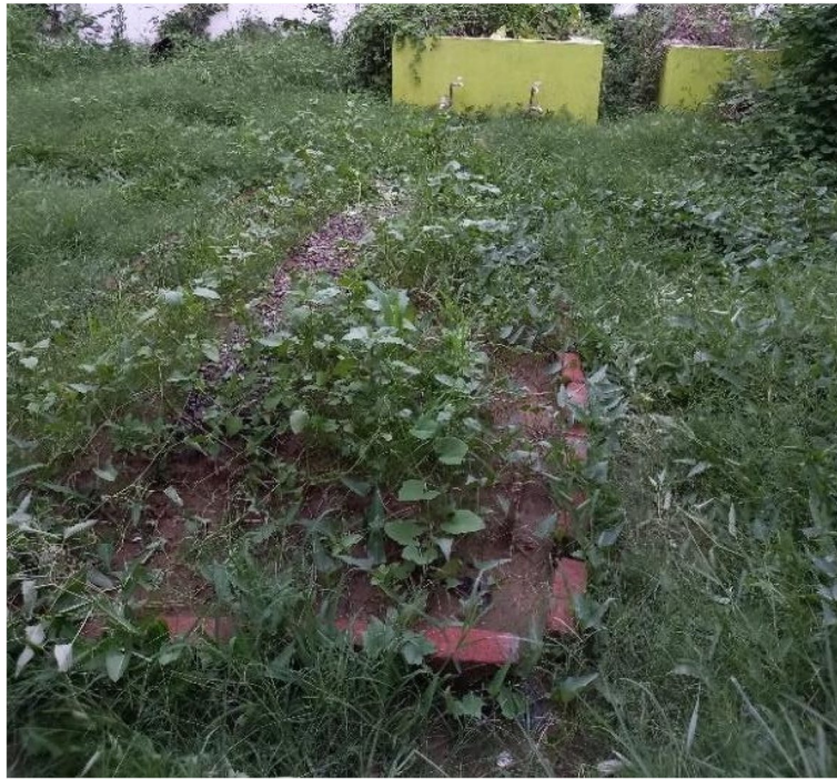
Fig. 19 Shows significant cover of vegetation over embankment
