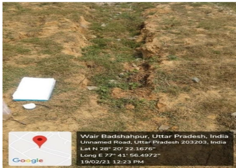
Fig. 4 Studied embankment at Wair, showing effect of gullying and slope failure no 2
