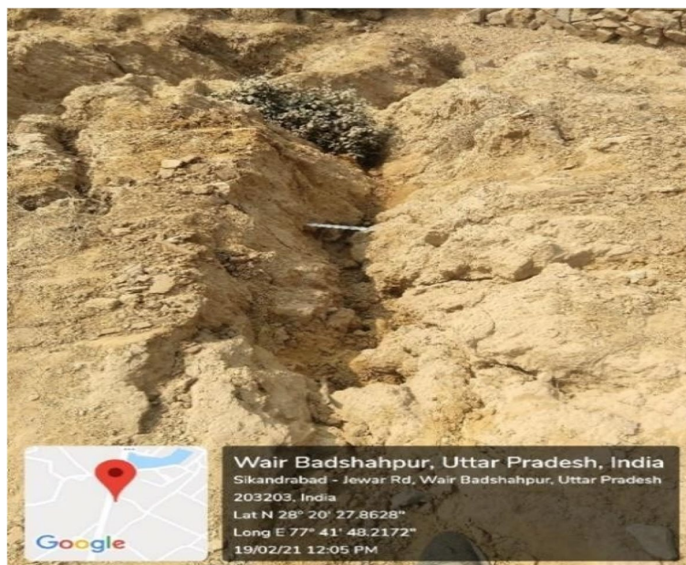
Fig. 3 Studied embankment at Wair, showing effect of gully and slope failure no 1
