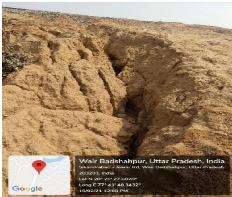
Fig. 5 Studied embankment at Wair, showing effect of gullying and slope failure no 3
